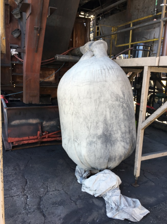
Dust collection and Enclosures
